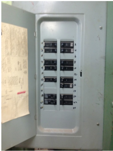
Figure 18. The Service Entrance Panel (SEP) and sub-panels house the circuit breakers for the AC circuits.
