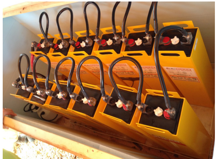
Figure 15. A bank of two strings of 2 volt batteries wired in series. Each string is 12 volts.
