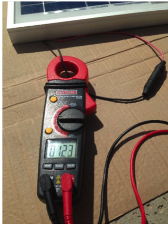
Figure 10. Measuring short-circuit current (Isc) with a clamp-on DC multimeter to check if the rated short-circuit current (Isc) value matches the specification sheet.
