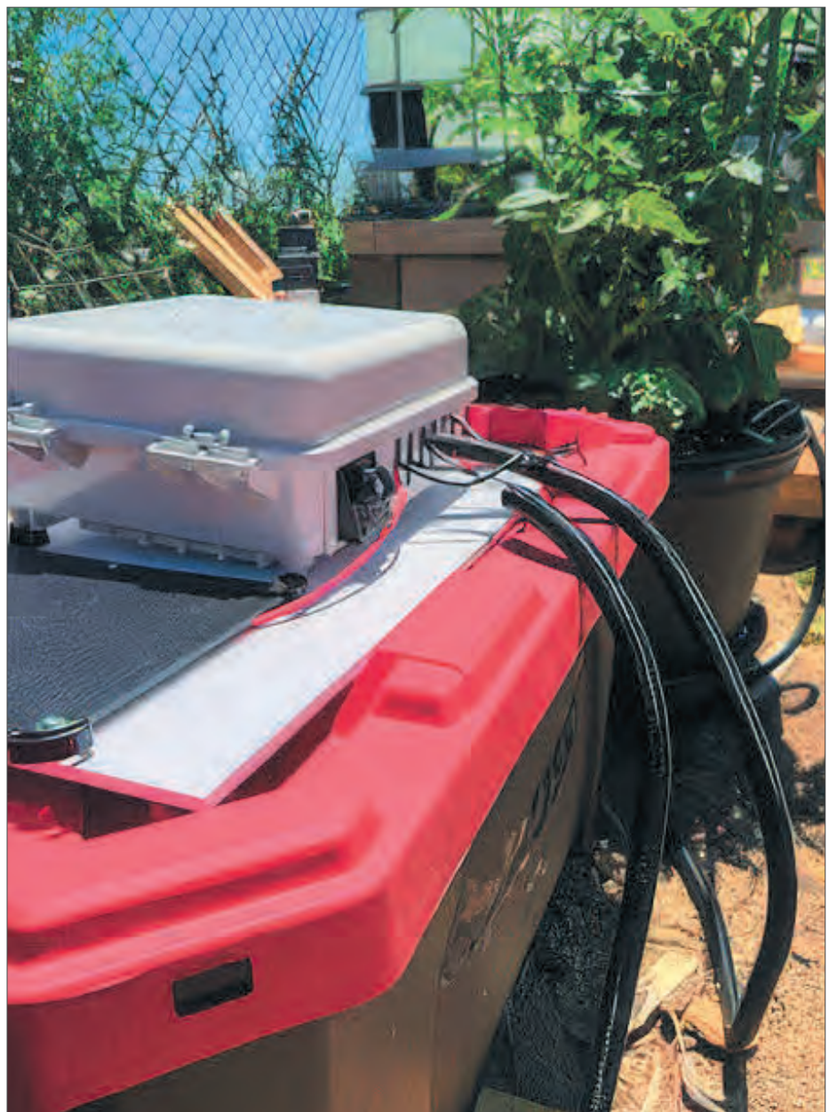
The control box sits at the heart of the AI demonstration.
