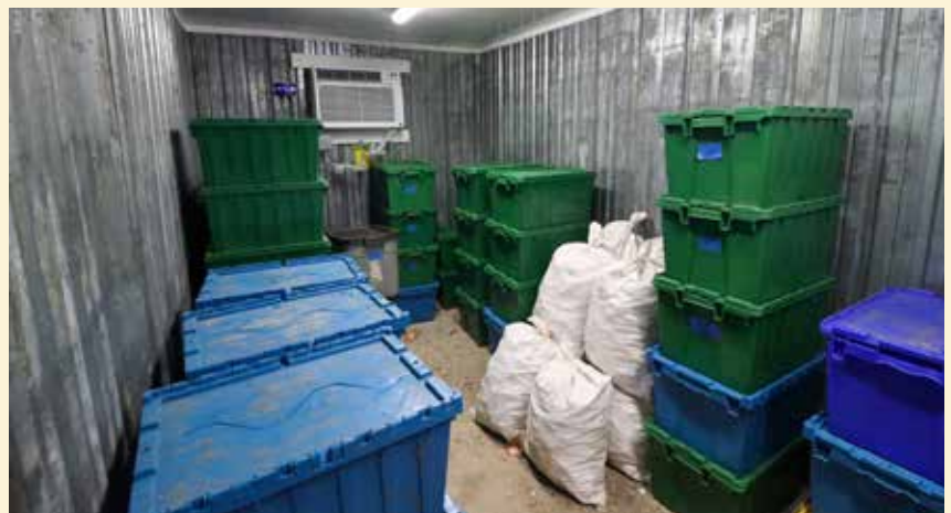
This storage shed uses low-heat lighting and a standard air conditioning unit connected to a CoolBot temperature controller. Photo by Andy Chamberlin, University of Vermont Extension
