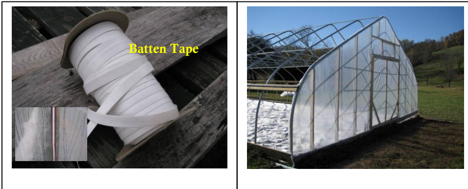
Figure 14. Batten tape is used to secure the plastic to the end wall frame.
