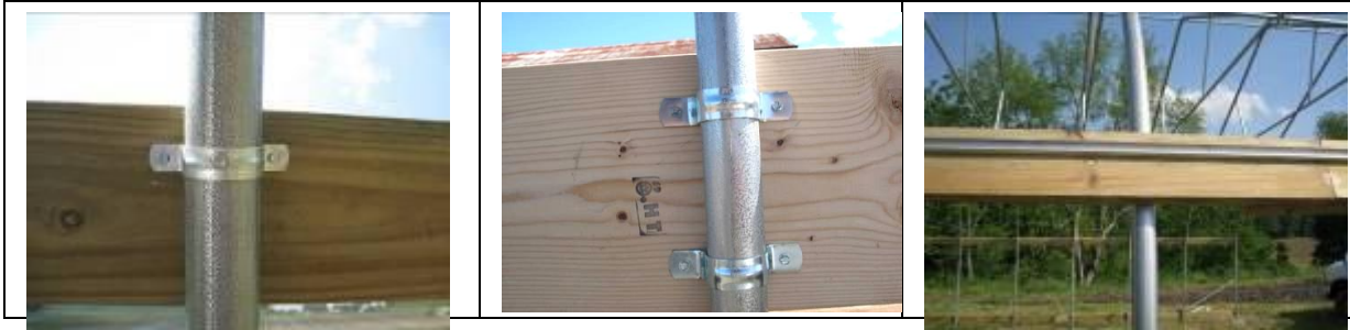
Figure 9. Pipe straps are used to secure the baseboards and hipboards to the high tunnel frame. Aluminum channel lock is used to secure the plastic to the frame.
