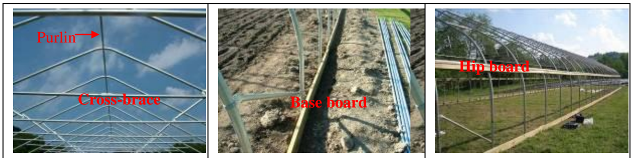
Figure 8. Purlins, cross braces, base boards and hip boards are attached to each bow to provide stability to the high tunnel frame.
