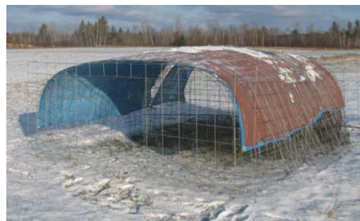
▲ Photo 2. The Day Range hoopie is an easy to build and sturdy structure that can be moved by one person and will last for many years. It will comfortably hold up to 150, 8-week chickens overnight.
