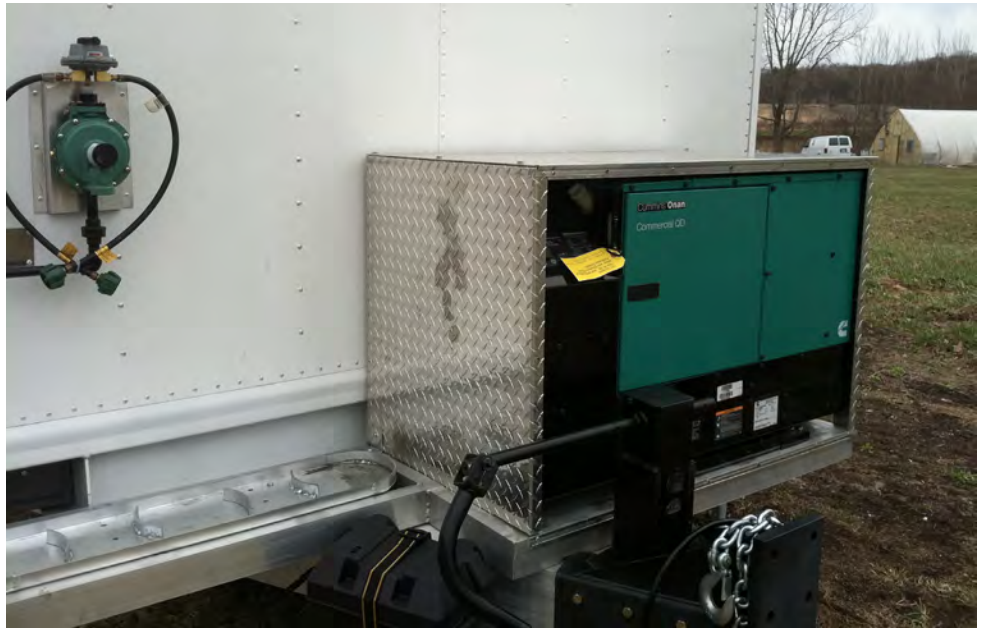
Propane connections and regulator (left), diesel generator on Massachusetts enclosed MPPU
