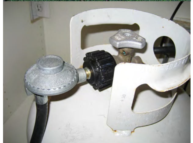
Top: Propane cylinders connected to regulator with changeover valve.
