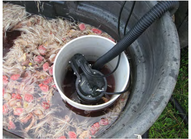
“Offal soup,” the product of mingling solid processing wastes with wastewater. Here a sump pump is sending the liquid waste to a compost pile, with a screen preventing (or attempting to prevent) the solid waste from clogging the pump.
