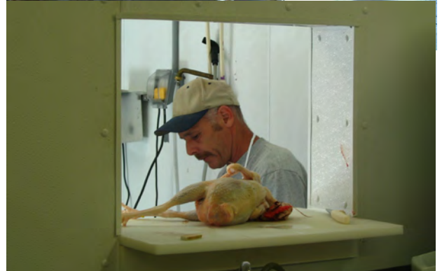
Top: Pass-through on enclosed Massachusetts MPPU, with kickout door from plucker Middle: Kickout door in action (a plastic “backstop” was later added to the catch table) Bottom: Pass-through window, Stone Barns Center
